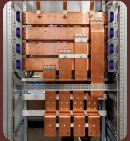
Power Panels S.A.
