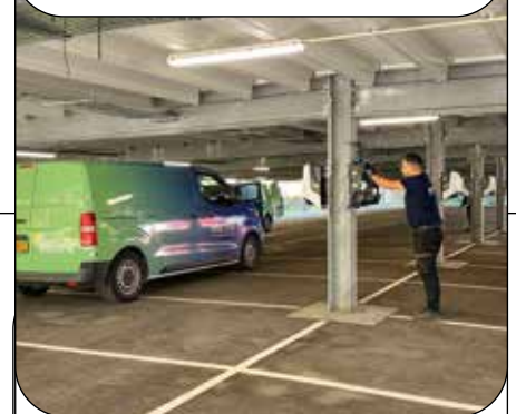
Borne de recharge parking / Parkplatz-Ladestation
