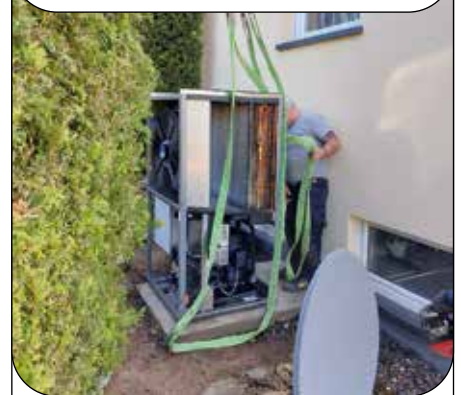
Installation PAC LuxProof
